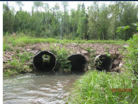
Valley Drive Culvert—Very Poor Condition-
